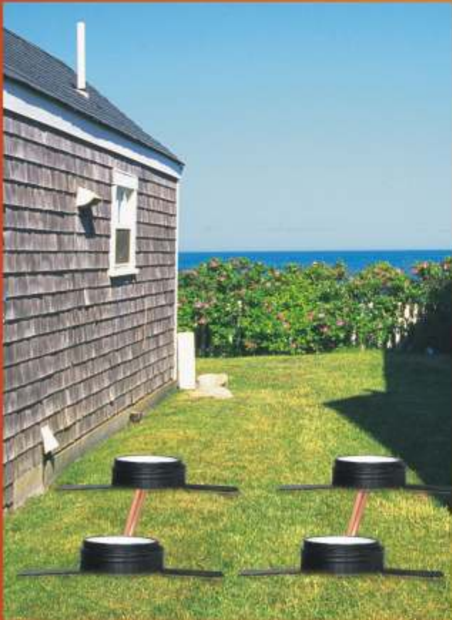
Inter connective tank
